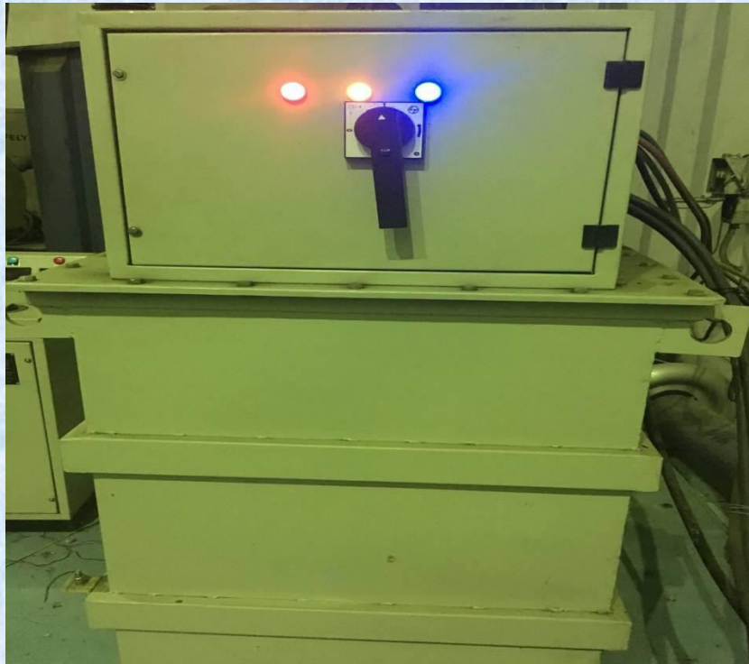
3-Phase Booster Transformer
